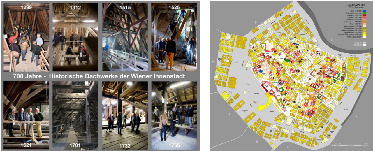
Fig. 1. The traditional roof structures in Vienna go back to the year 1299. These findings from the Middle Ages can be studied during very rare guided tours and they regularly arise enthusiasm and great interest among the public (© Bettina Neubauer-Pregl, Katharina Steudtner, Michal Panáček).
