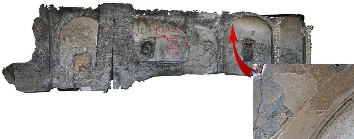
Fig. 8. Remains of a stuccoed vault in a room of the northern facade of the pars maritima, probably used as a triclinium. Screenshot of 3D model (© W. Filser, B. Fritsch)
