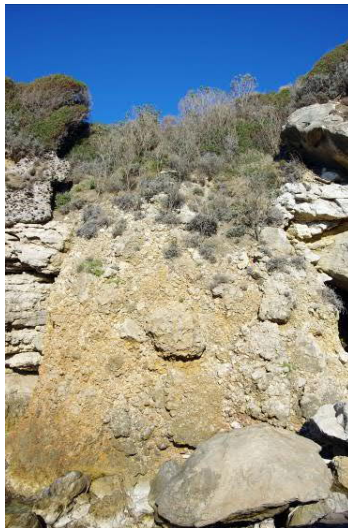
Fig. 15. Rockslide seen from the outer harbour (west) (© M. Reinfeld)
