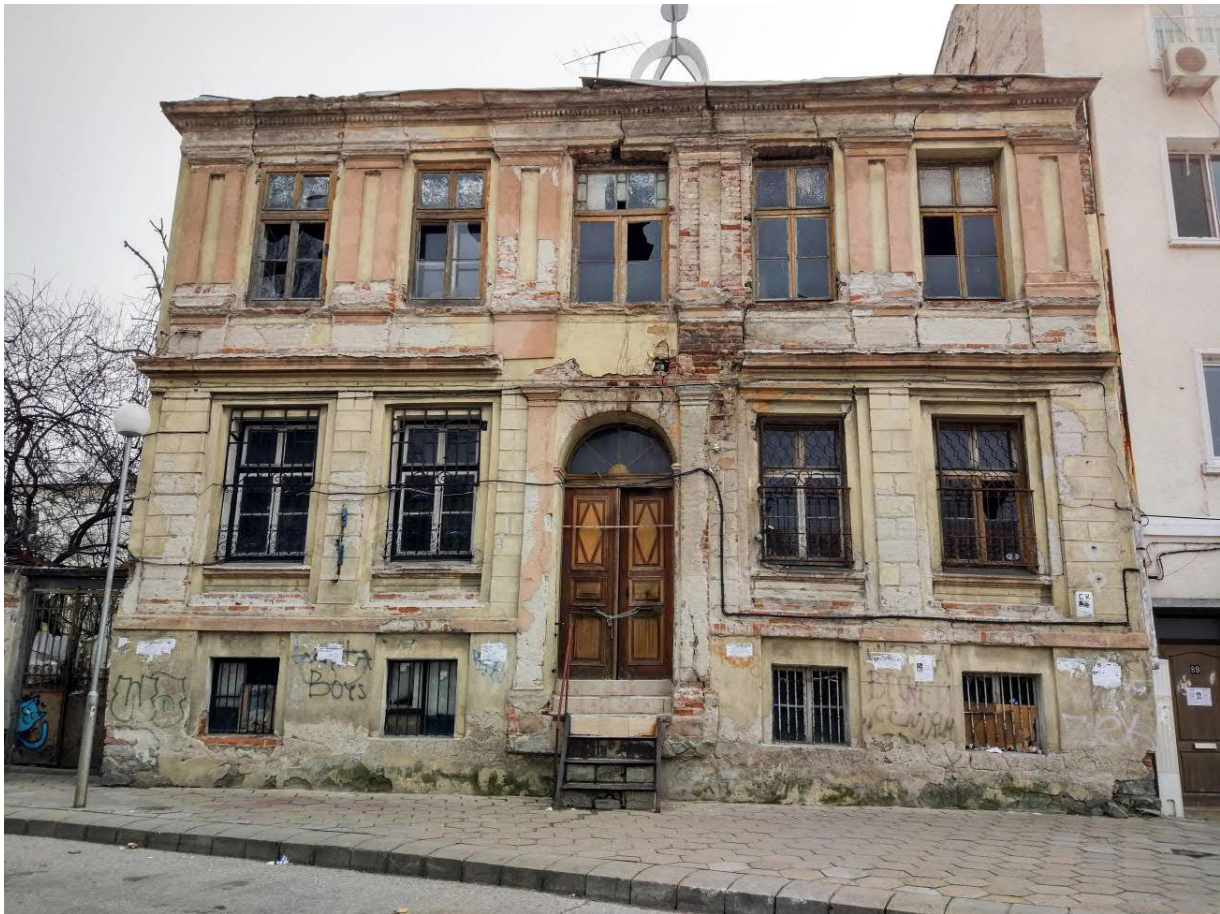
Fig. 6. Monument in decay, © N. Toleva-Nowak
